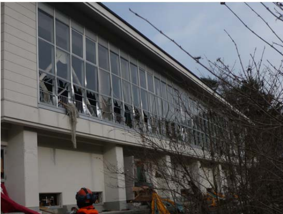
Gymnasium in Japan 12m above sea level – note the fishing nets coming out the windows
